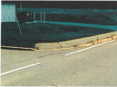
Curb ramp with cracks
