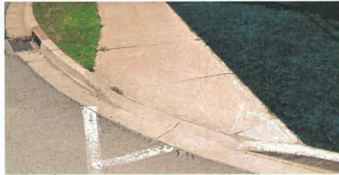
Curb ramp wider than the curb edge
