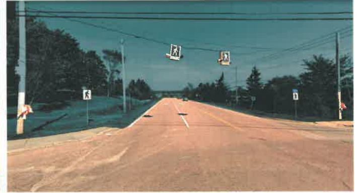
Crossing at HW2 with flags, markings, and push button
