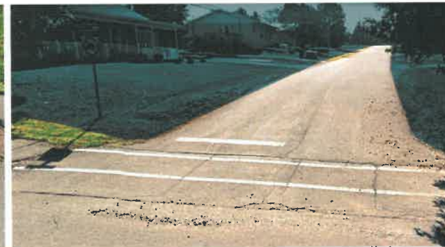
Narrow crosswalk with no signage on either side
