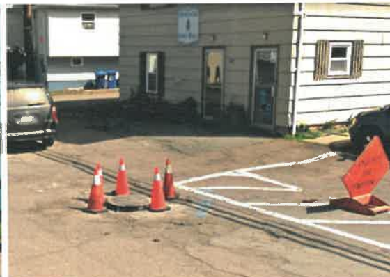
Unpaved sidewalk near Town Hall and library
