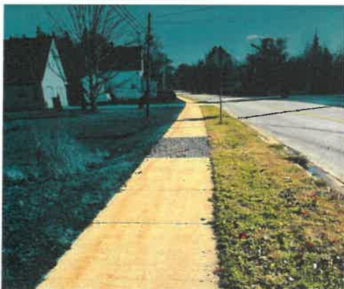
Gravel patch in between concrete paving
