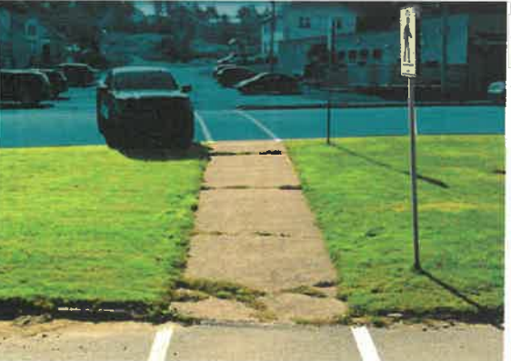
Median crossing with uneven surface
