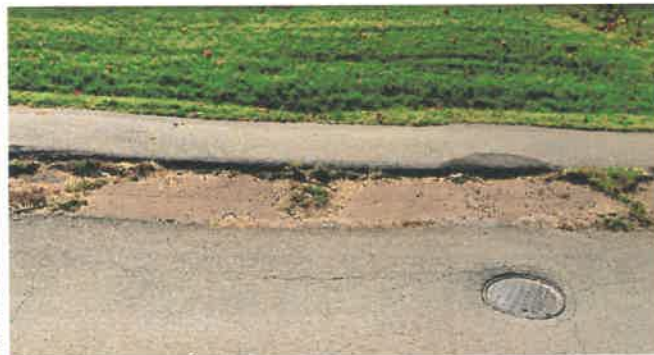
Uneven surface with sunken paving and large cracks
