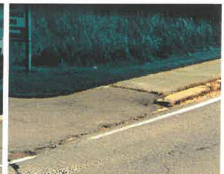
Uneven surface and withered curb edges
