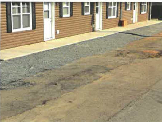
Unpaved hazard prone path on one side of the road
