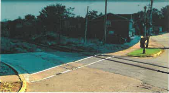
Narrow crosswalk with uneven surface
