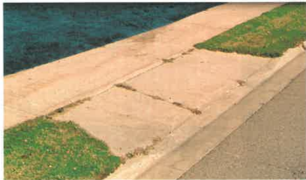
Growing grass in between concrete slabs on civic curb ramp
