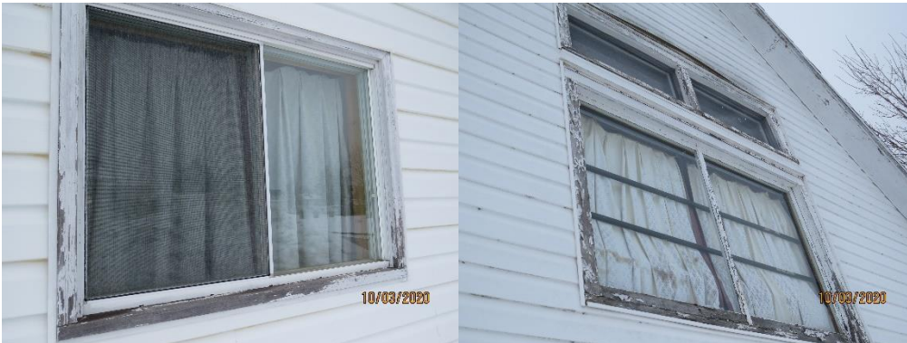
Wood windows in fair condition- will require replacement in future
