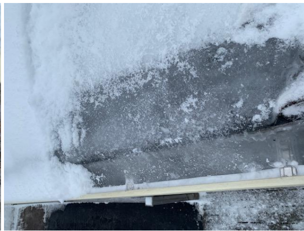
ice dams at gutters and downspouts
