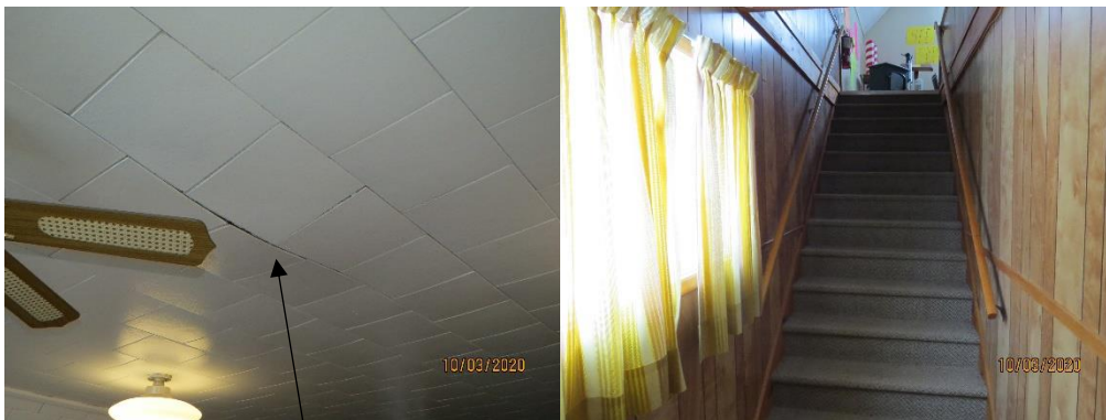
Upper floor ceiling- minor damage
