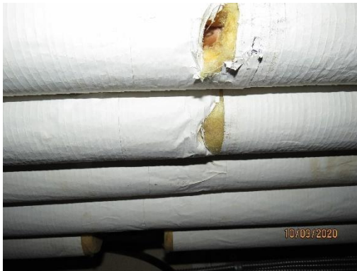
Poorly insulated piping
