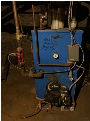
Boiler installed year 2000
