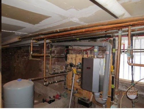
Natural gas heating system
