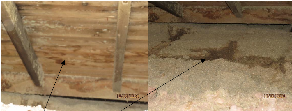
Attic space evidence of water leaks
