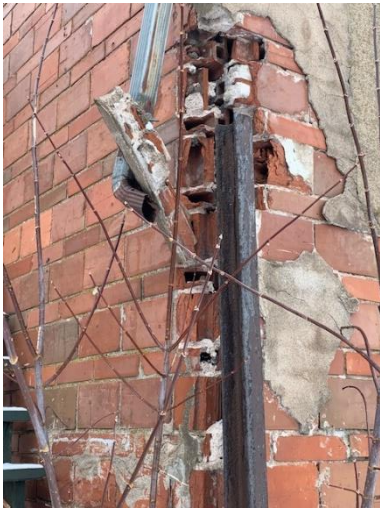
Exterior masonry failing
