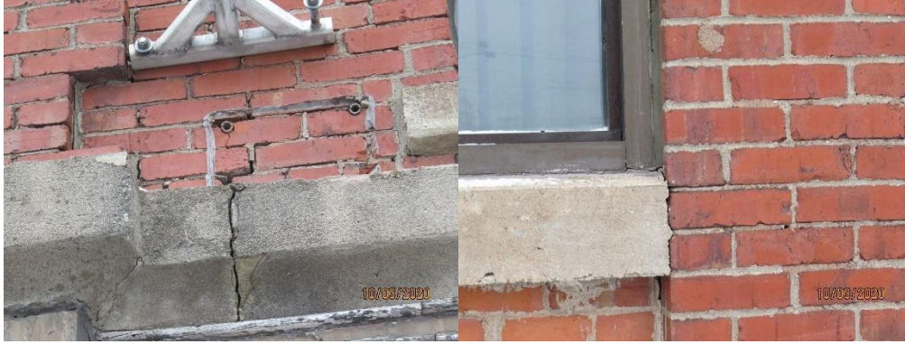
Front elevation, structural deflection and cracking
