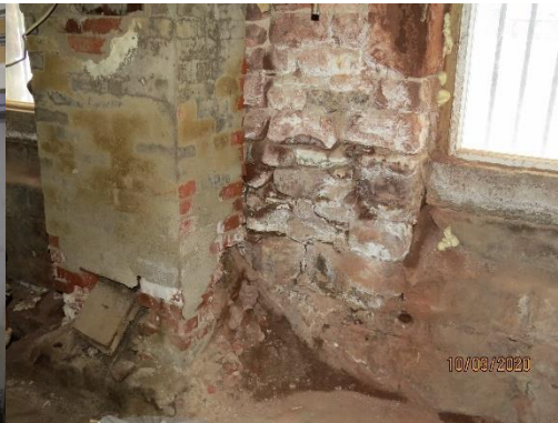
Structural decay at former chimney
