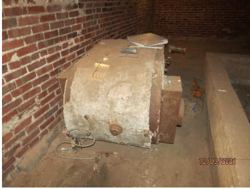
Old boiler in basement- likely asbestos
