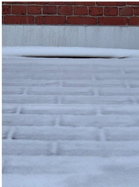
flashing detail not sealed
