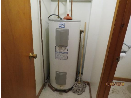
1989 domestic hot water tank
