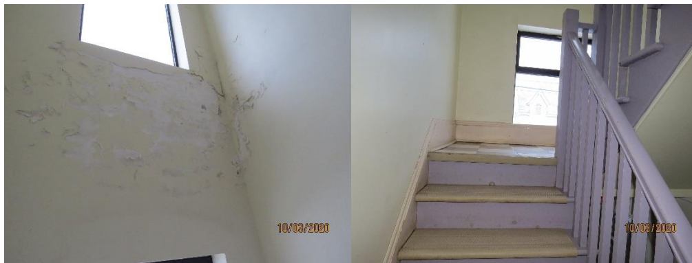
Stair system with extensive paint peeling
