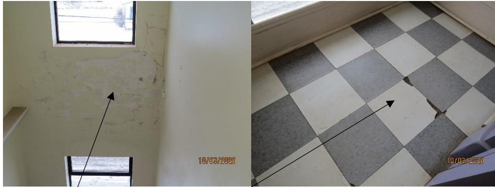
Going upstairs- paint peeling and floor damage
