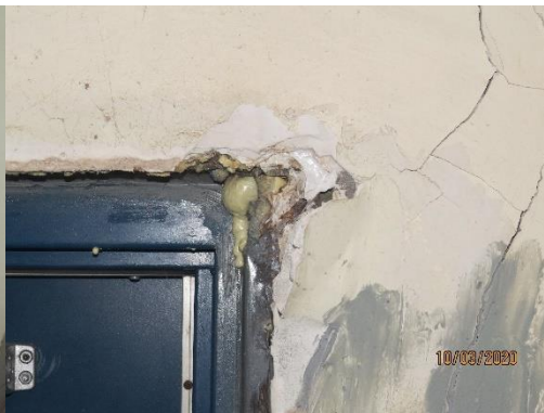
south door frame and substrate decay
