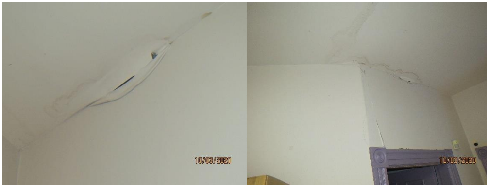
Evidence of moisture leakage
