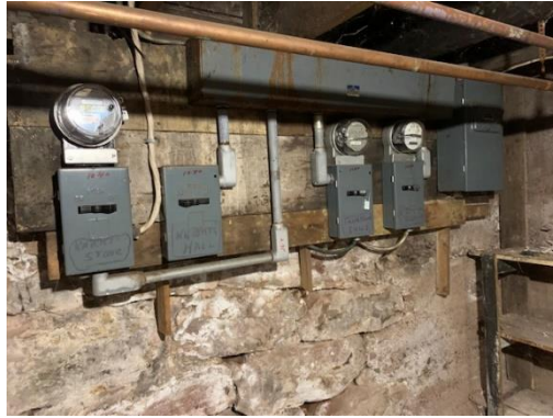
Main electrical service in basement- rust and water stains
