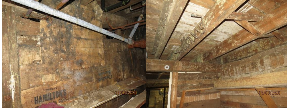
Basement areas with extensive mould evident
