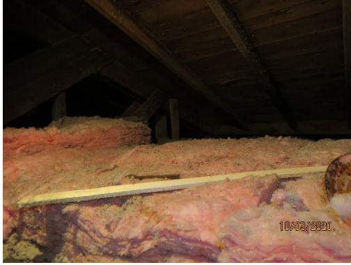
Attic space water leaks
