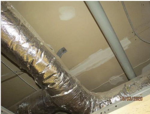
Upper floor ventilation- minimal air flow
