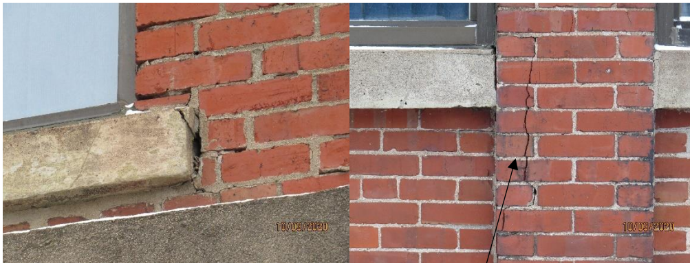
Front elevation masonry cracks and missing mortar- stress cracking
