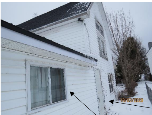
Wood windows cladded in aluminum- unknown condition. Rear elevation door in fair condition.
