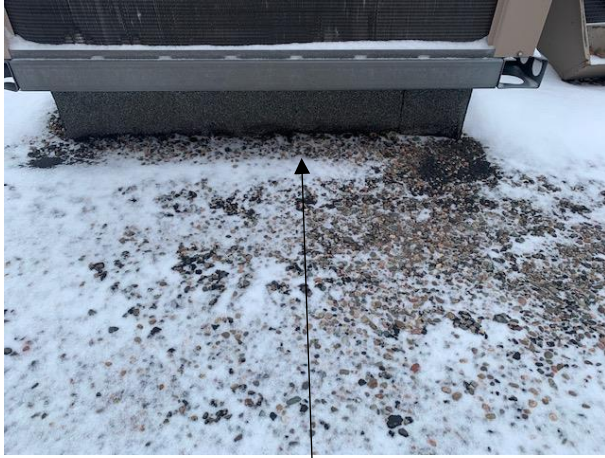
Roof decay at HVAC unit
