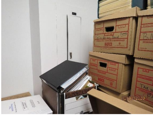
Electrical panel blocked in records storage Code violation
