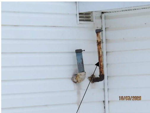
Fuel tank lines. Vent shall extend a minimum 2' above any building opening or roof line. Code issue.
