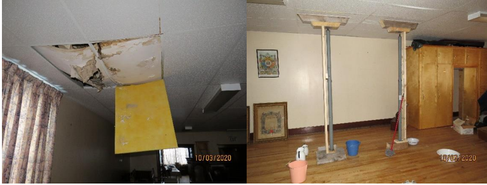
Upper floor ceiling collapse due to roof leaks- mould evident
