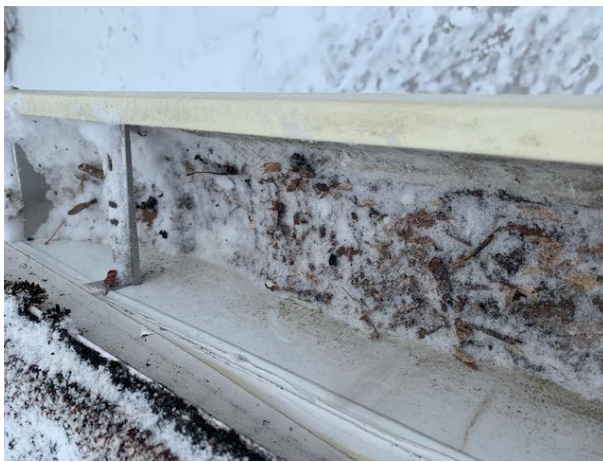
eavestrough full of debris
