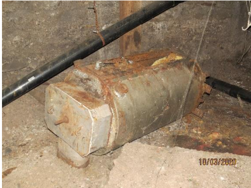
Old boiler in basement-likely asbestos
