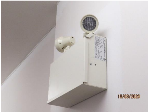
Emergency lights not working
