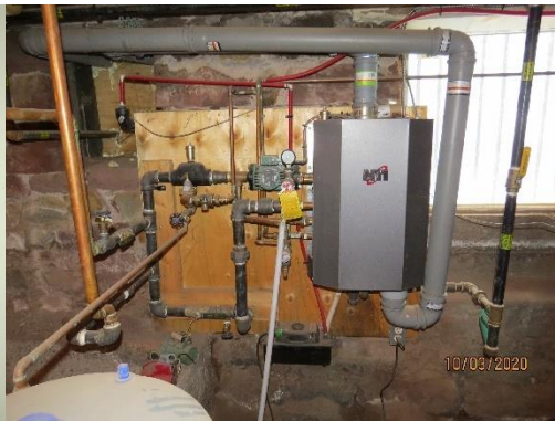
main heating system- pipes not insulated
