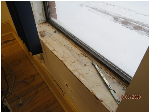
Evidence of moisture issues
