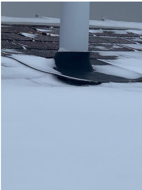
Plumbing vent not sealed
