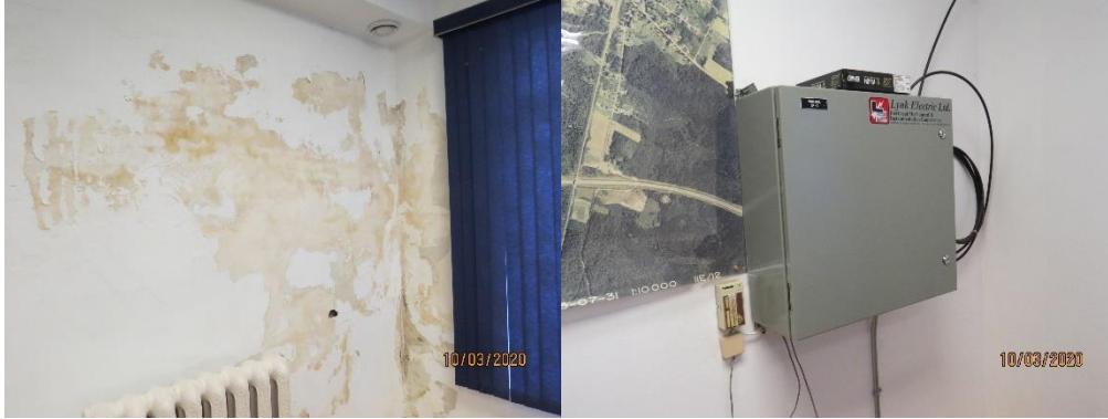
Moisture leakage evident
