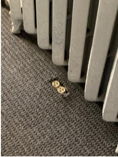
Electrical in floor not to Code
