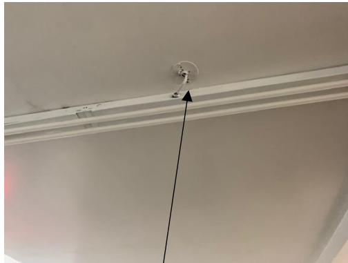
interior lighting-wiring not to Code
