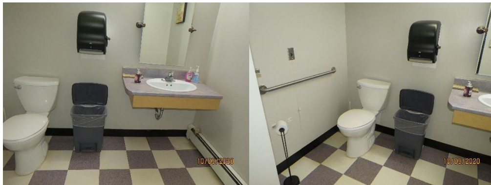
Main floor bathroom does not meet NBC section 3 and BF 651 Barrier Free standards
