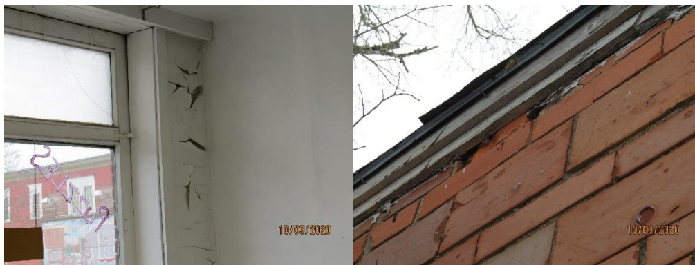
Front entry window leaks
