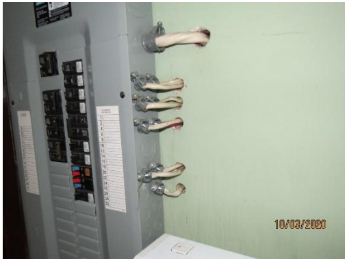
Electrical panels not to Code
