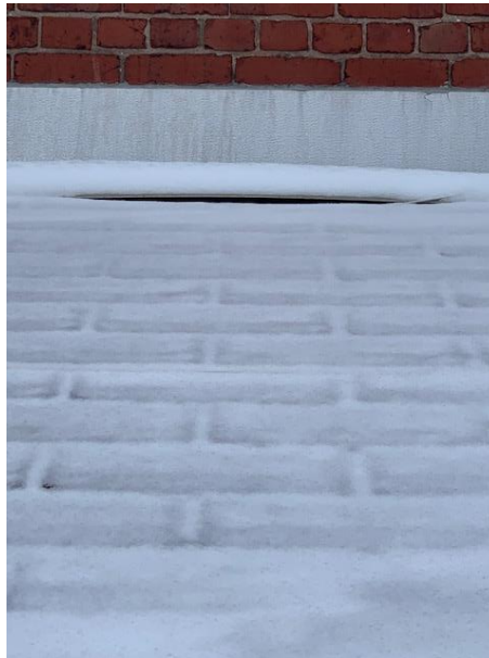
flashing detail not sealed
