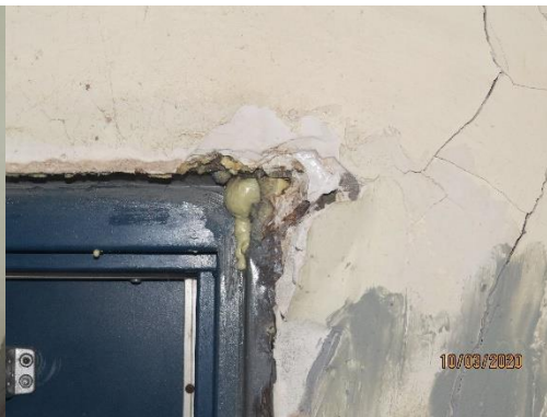
south door frame and substrate decay
