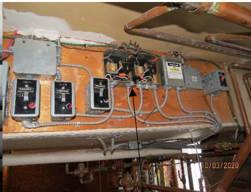
Code violations- open electrical boxes
