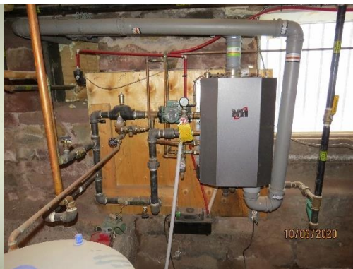
main heating system- pipes not insulated
