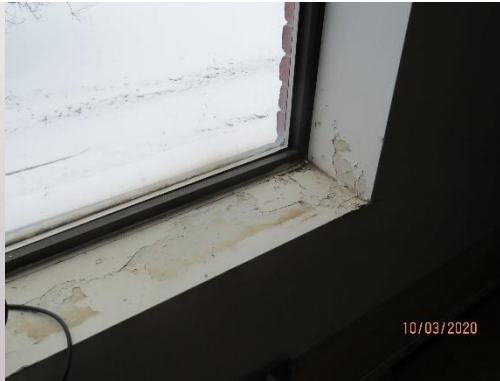
Extensive moisture at windows
