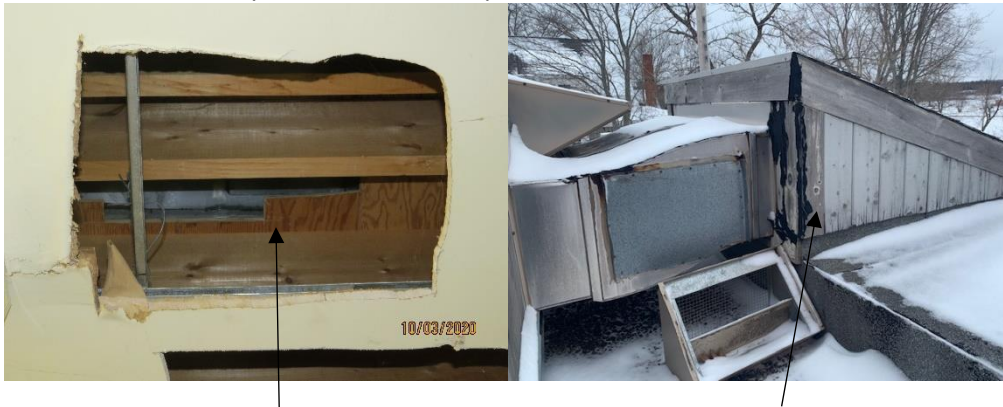
Main hall near safe, roof leak, likley source is the roof ventilation duct work not properly sealed
