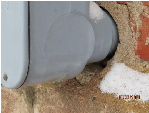
Wall penetrations for electrical not sealed
