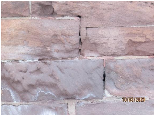
Masonry and stone damage
