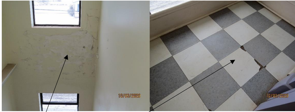
Going upstairs- paint peeling and floor damage
