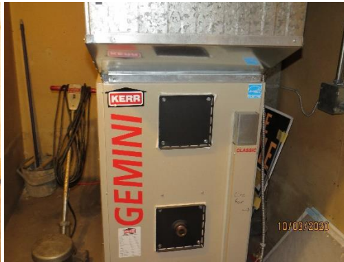
oil fired heating furnace
