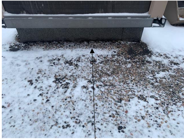
Roof decay at HVAC unit
