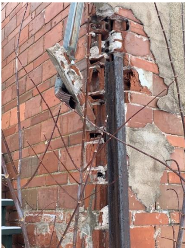
Exterior masonry failing
