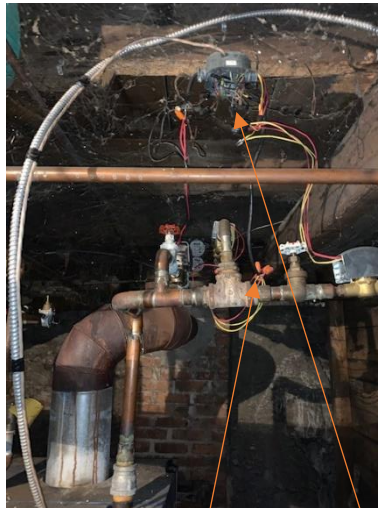
Open electrical devices not to code
