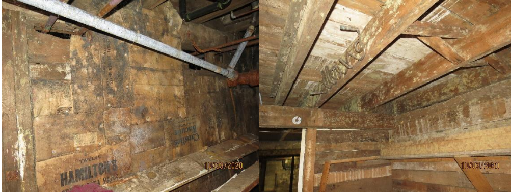
Basement areas with extensive mould evident
