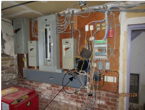
Electrical code violations
