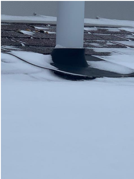
Plumbing vent not sealed
