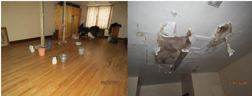
Water collection buckets for roof leaks
