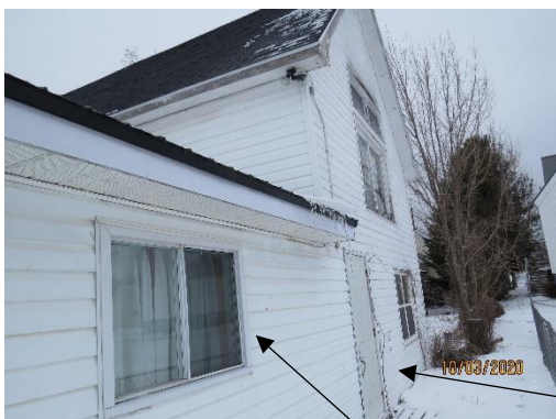
Wood windows clad in aluminum- unknown condition. Rear elevation door in fair condition.
