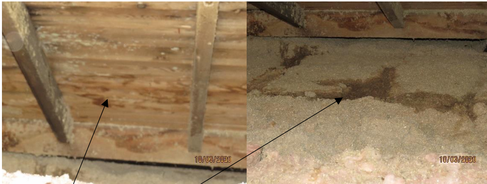
Attic space evidence of water leaks
