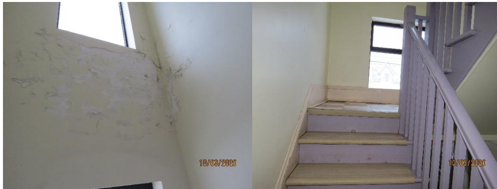
Stair system with extensive paint peeling
