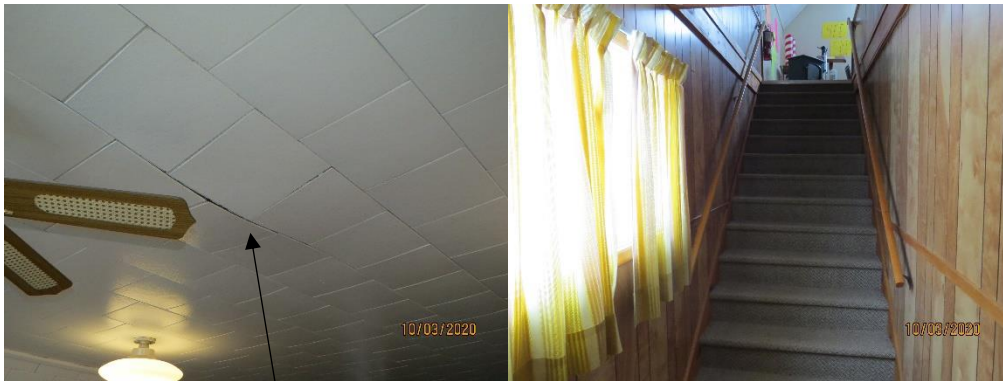
Upper floor ceiling- minor damage
