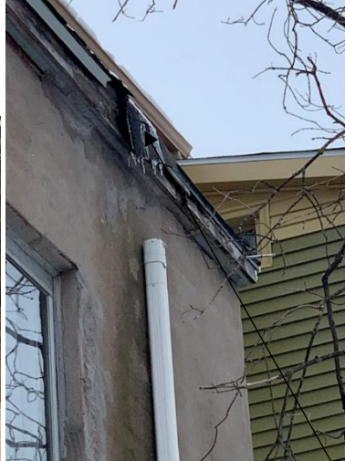
Roof shingle system sliding off roof-failing
