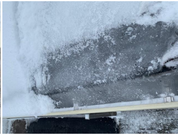
ice dams at gutters and downspouts
