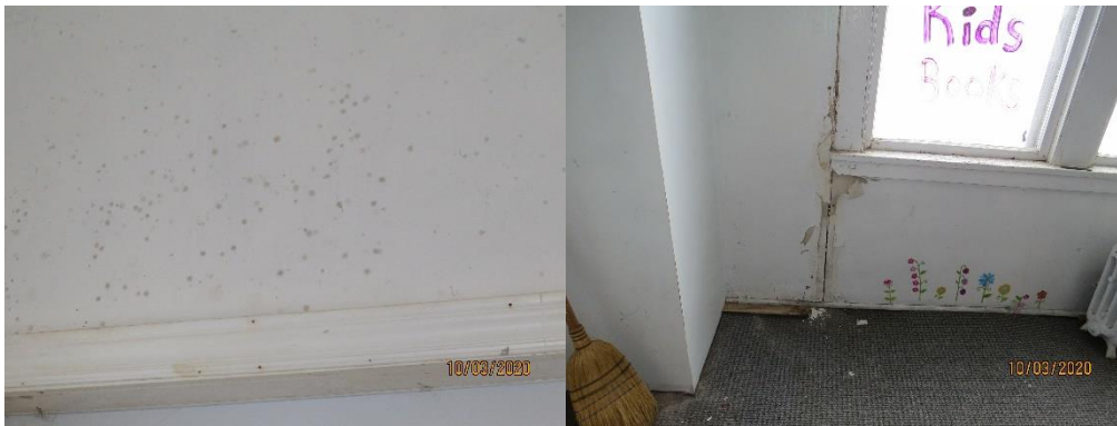
Main floor rear exit with mould on walls
