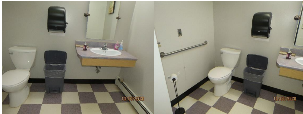
Main floor bathroom does not meet NBC section 3 and BF 651 Barrier Free standards
