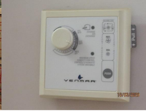
Air/humidity controller set at minus 10 degrees However system indicator lights (activity) not on.
