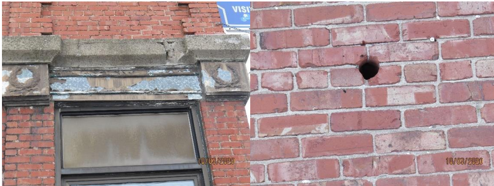
South elevation masonry decay and approx. 2" hole
