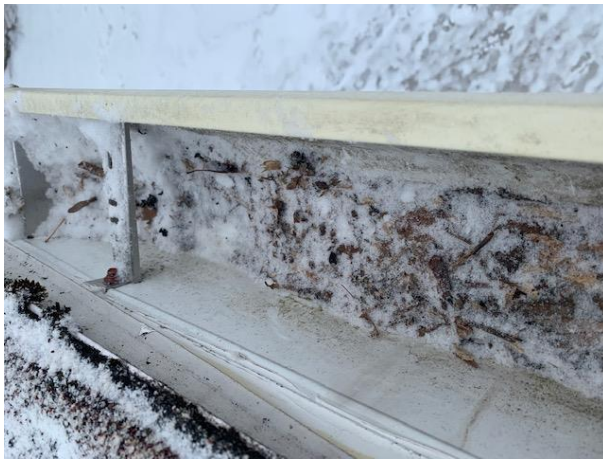
eavestrough full of debris
