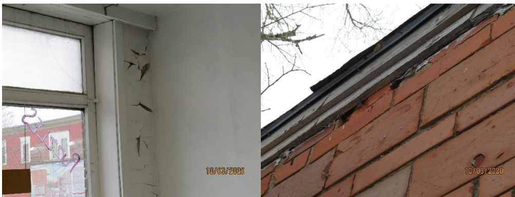
Front entry window leaks
