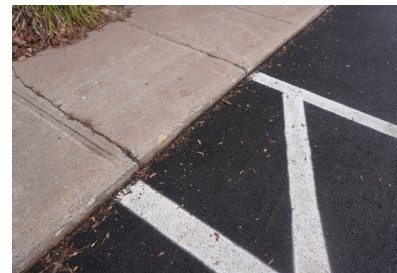
Crosswalk connected to sidewalk curb (no curb ramp).
