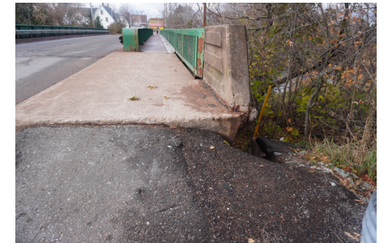
Drop-off at Water St. bridge.
