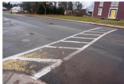
Painted crosswalk across Main St. with white lines and faded yellow.
